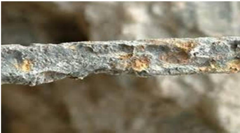
FIG.1: CORROSION IN REINFORCEMENT
