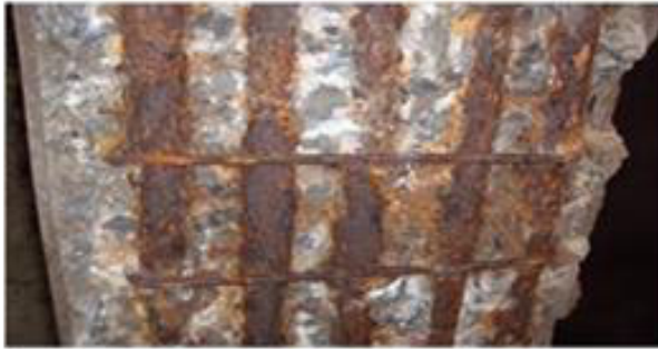
FIG.2 CORROSION IN RC STRUCTURE
