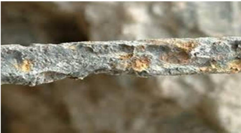
FIG.1: CORROSION IN REINFORCEMENT
