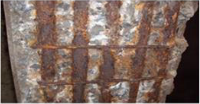
FIG.2 CORROSION IN RC STRUCTURE
